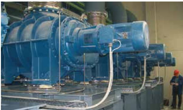
4-stage vacuum plant with 2 x 30,000 m 3 /h intake volume flow in steel degassing
