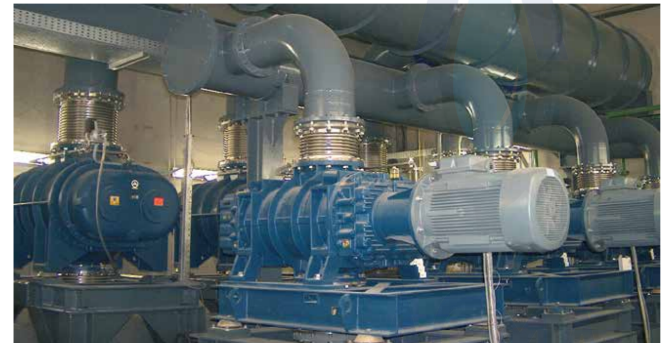
4-stage vacuum system with 2 x 30,000 m³/h intake volume in steel degassing
